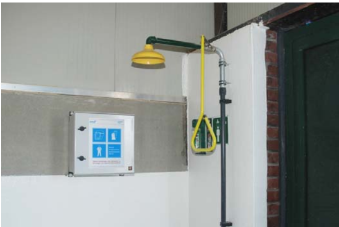
Figure 3-4: Emergency shower and safety cabinet
