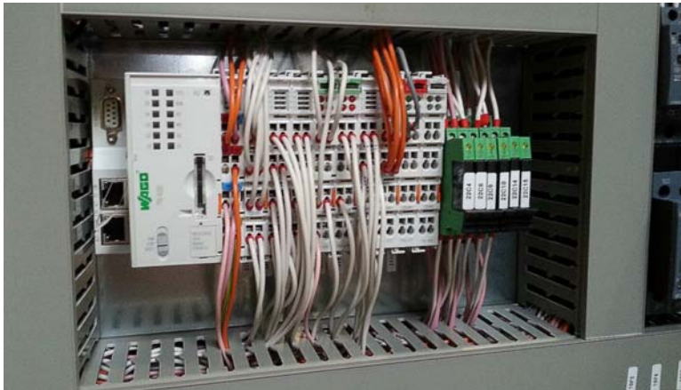
Figure 7-2: Data logger with SD card in the control cabinet
