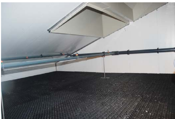
Figure 4-2: Filter package with sprinkler pipe
